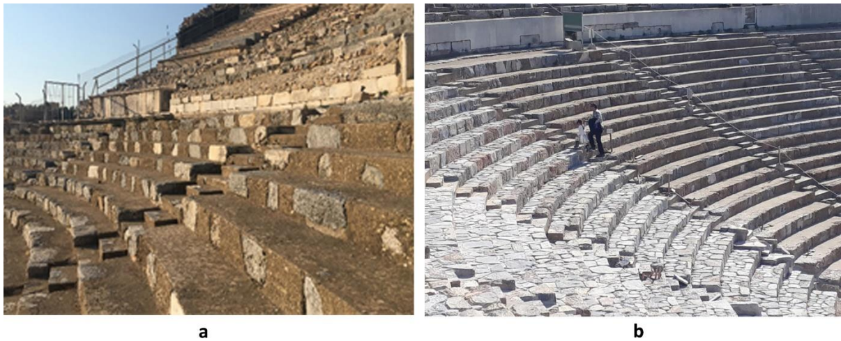
Figure 2. a.Repairs with cement-based mortar and concrete completions made in the 70s (Republic of Türkiye Ministry of Culture and Tourism, 2021), .b.The difference in texture of the completions with hydraulic-lime-based mortar and stones carried out during works between 2019-2021 and the parts with cement repairs made in the 70s (Yılmaz, 2019-2021)
