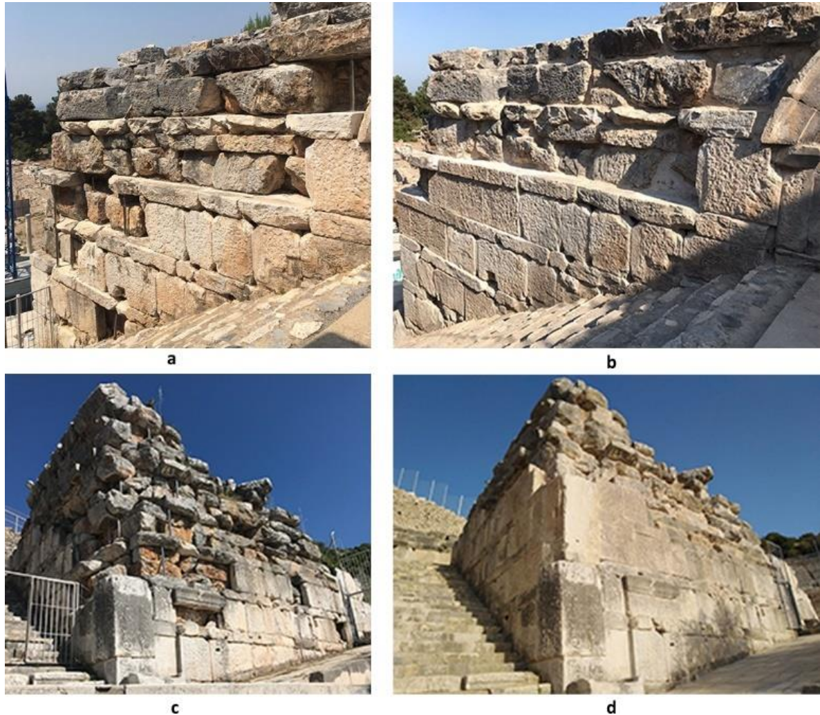
Figure 7. a. Sample of the reinforcement works on the Parodos walls, stones supported with metal poles (Yılmaz, 2019-2021). b. Partial stone completion during reinforcement and strengthening works between 2018-2021 (Yılmaz, 2019-2021). c. Wall stones supported with metal poles (Yılmaz, 2019-2021). d. Partial stone completion during reinforcement works between 2018-2021 (Yılmaz, 2019-2021)
