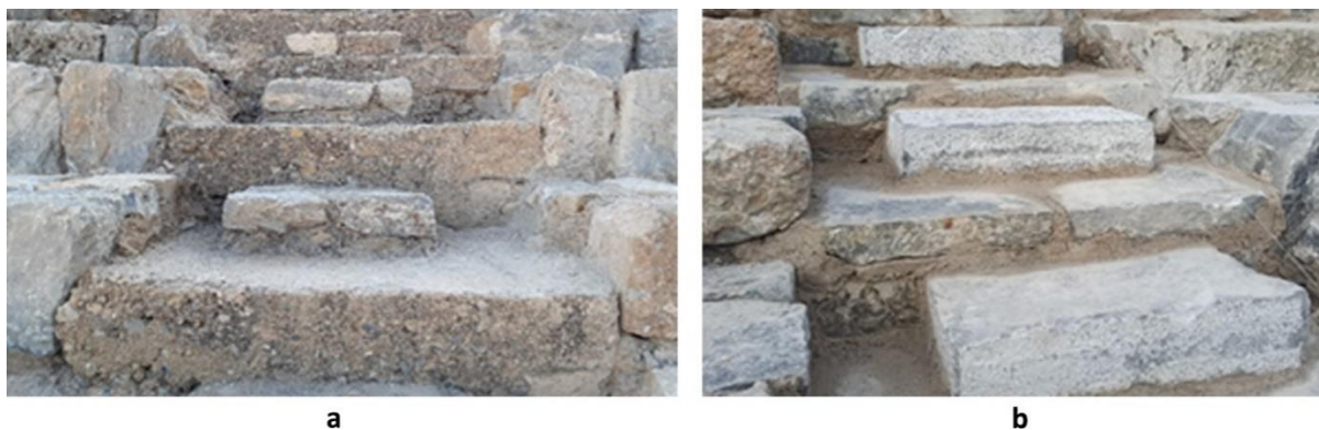
Figure 4. a. Concrete steps with cement repairs made in the 70s (Republic of Türkiye Ministry of Culture and Tourism, 2021), b. Steps formed with freestones during the works between 2018-2021 (Yılmaz, 2019-2021)
