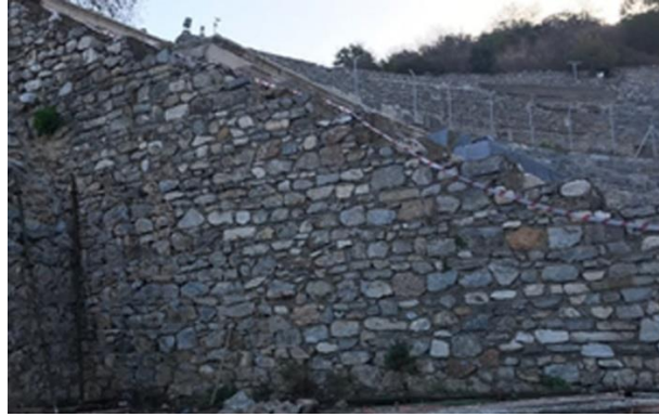
Figure 5. Reinforcement works carried out on the M4 Cavea substructure in the 70s. (Republic of Türkiye Ministry of Culture and Tourism, 2021)
